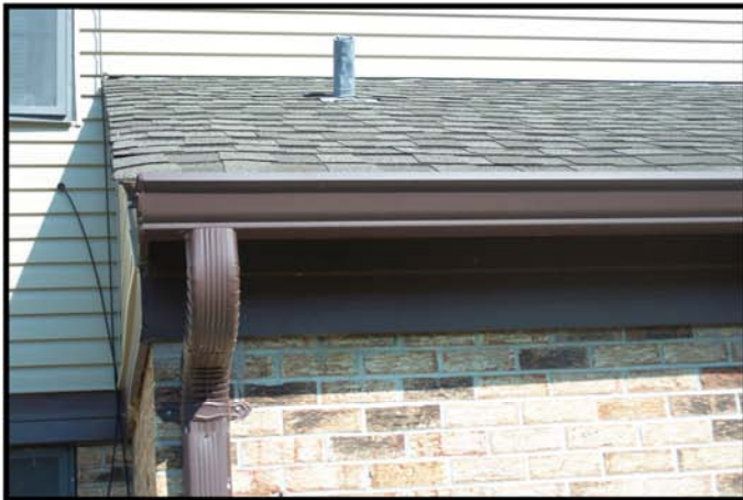
Replaced siding and fascia boards at Waltersville Estates (September 2011), Vicksburg Housing Authority.
