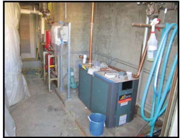
New electrical and HVAC systems (January 2012), Sacramento Housing and Redevelopment Agency.
