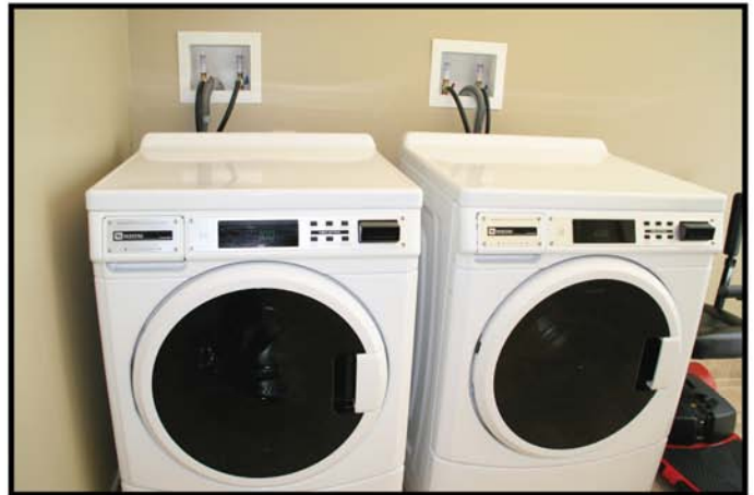
Renovated laundry room at Chishire Bridge High Rise (December 2011), Atlanta Housing Authority.
