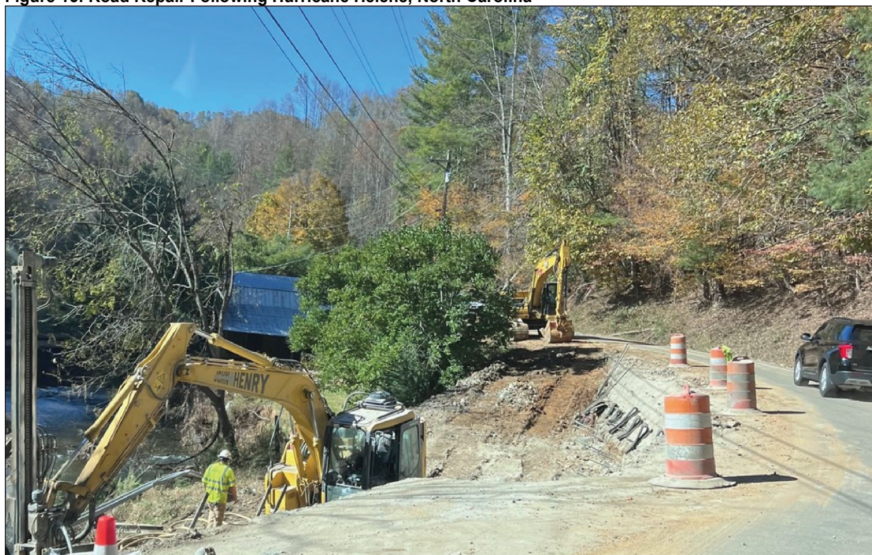
Figure 16: Road Repair Following Hurricane Helene, North Carolina
