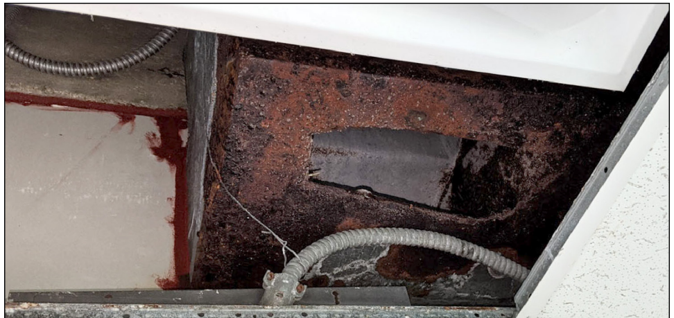
Figure 7: Corroded Outside Air Ductwork at Guam Memorial Hospital
