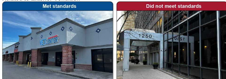
Figure 5: Examples of Readjustment Counseling Service (RCS) Inspection Findings Related to Exterior Condition
