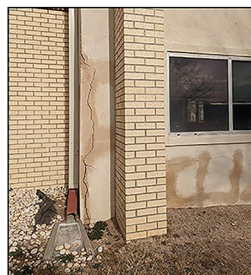
Residence facility in need of repair
