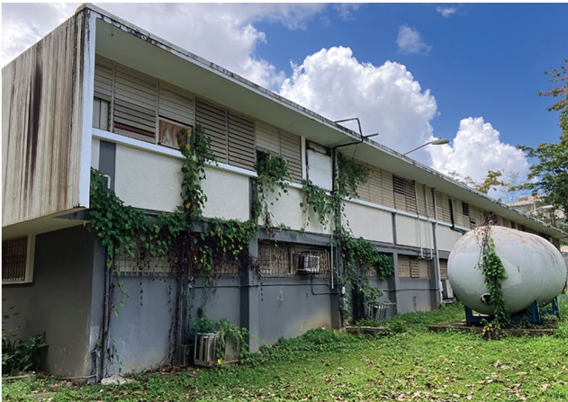
Medical building that was damaged by the hurricane in 2017 and has not been occupied since.
