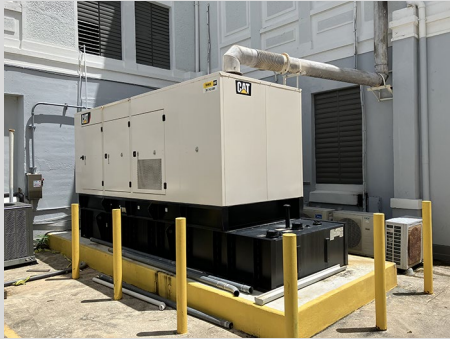
Generators purchased by an HSI to ensure continuity of operations.
