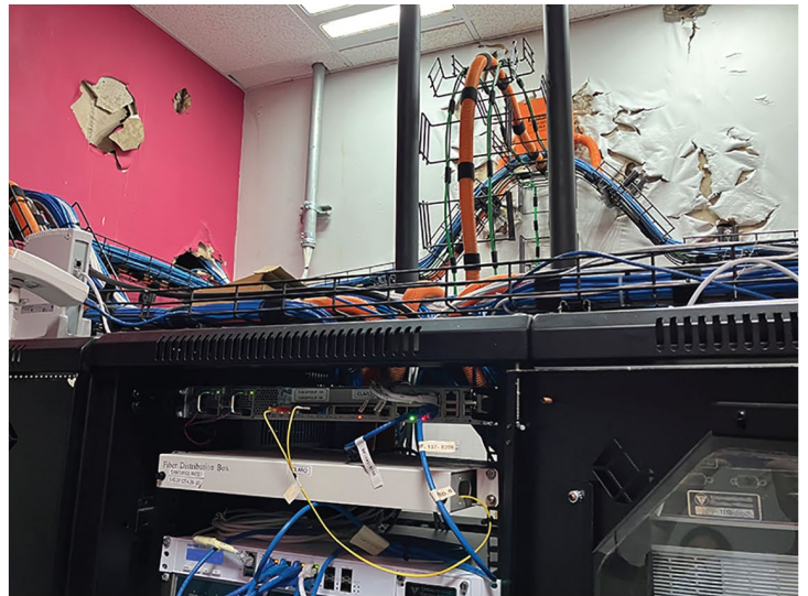
Damage in a server room sustained from the hurricane.
