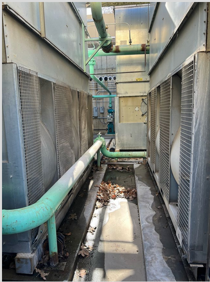
Above, these aging cooling towers are reaching the end of their lifecycle (about 25 years) and are critical to operating campus facilities.
