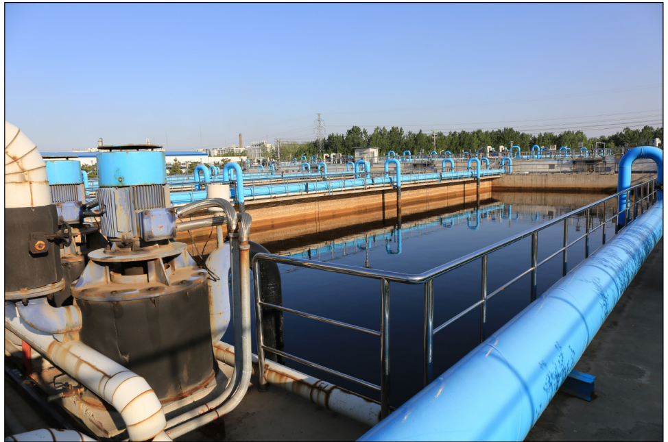
Figure 2: Example of Water System Pipes, Pumps, and Tanks That Could Be Monitored or Controlled by Operational Technologies
