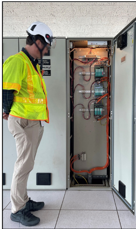
Figure 4: Examples of Water and Wastewater System Control Panels Containing Operational Technology Components
