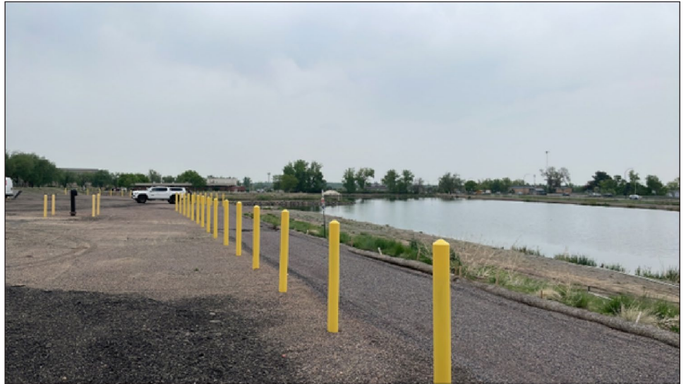
Figure 6: Reservoir with Interceptor Trench for Long-Term Treatment of Contaminated Groundwater at the Denver Federal Center, Lakewood, CO
