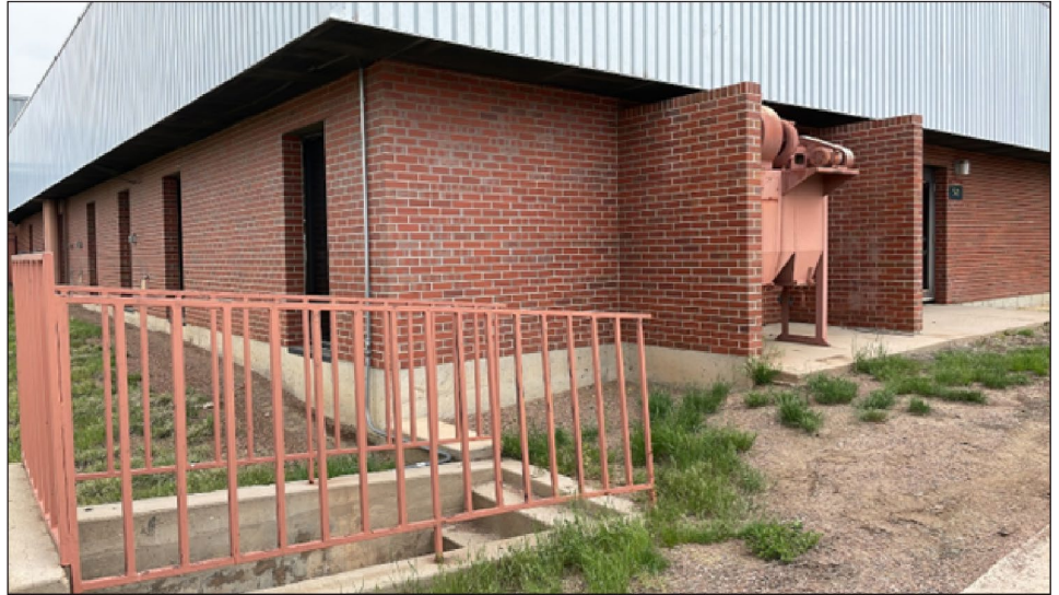
Figure 7: Building with Asbestos-Containing Materials that Is Scheduled to Be Demolished to Accommodate Future Development, Denver Federal Center, Lakewood, CO
