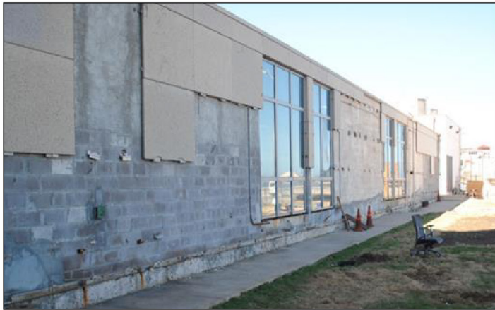
Damage to exterior walls.
