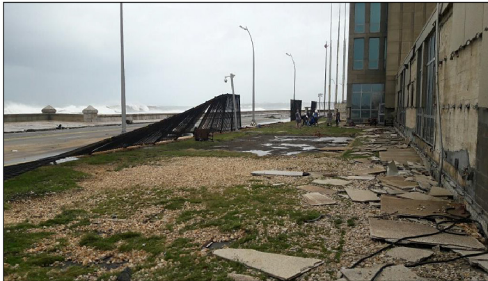
Damage to perimeter fence.
