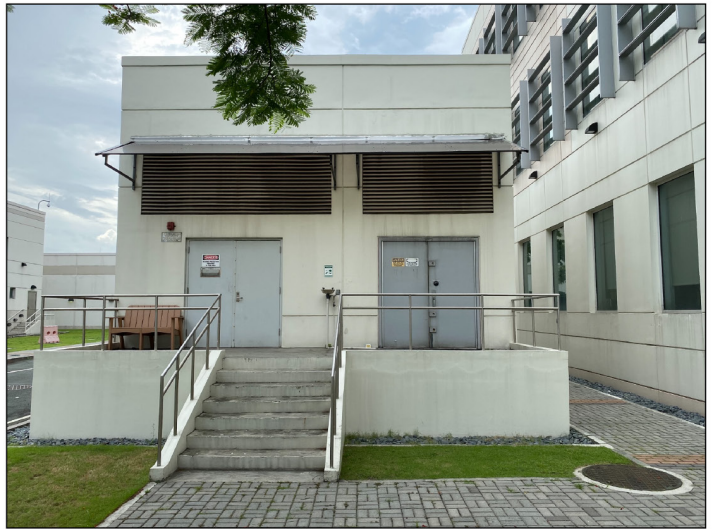
Chancery generators relocated and elevated.
