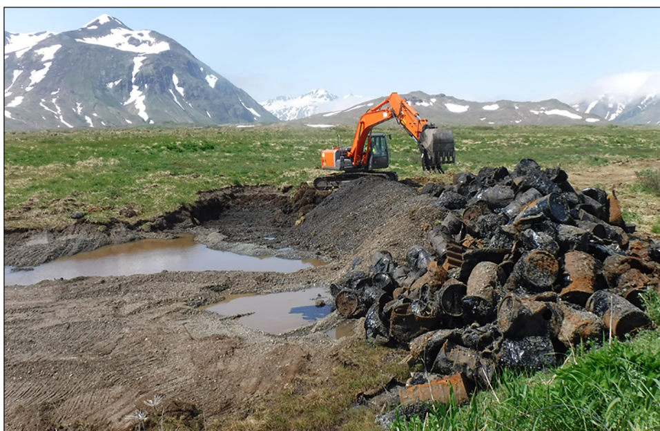
Figure 3: Department of Defense (DOD) Removal of Rusting and Leaking Barrels and Above-Ground Storage Tanks Threatening Migratory Birds on Attu Island
