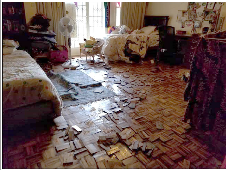
Figure 8: Damage to Post Housing in Kenya from a Water Leak
