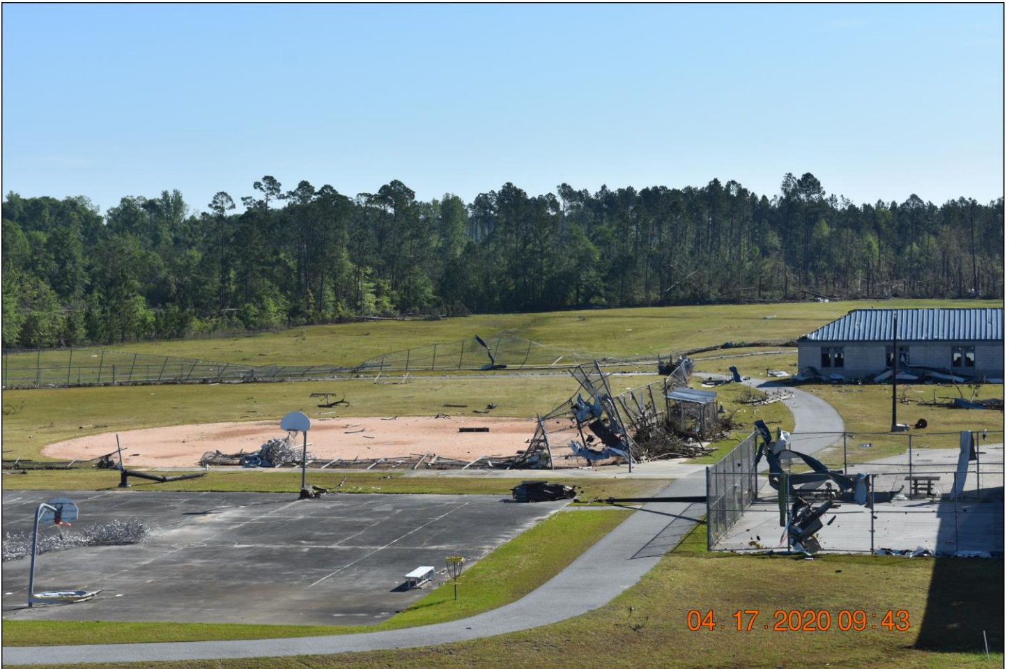
Figure 4: Tornado Damage to Perimeter Fencing and Recreation Yard at Federal Correctional Institution Estill in South Carolina, April 2020
