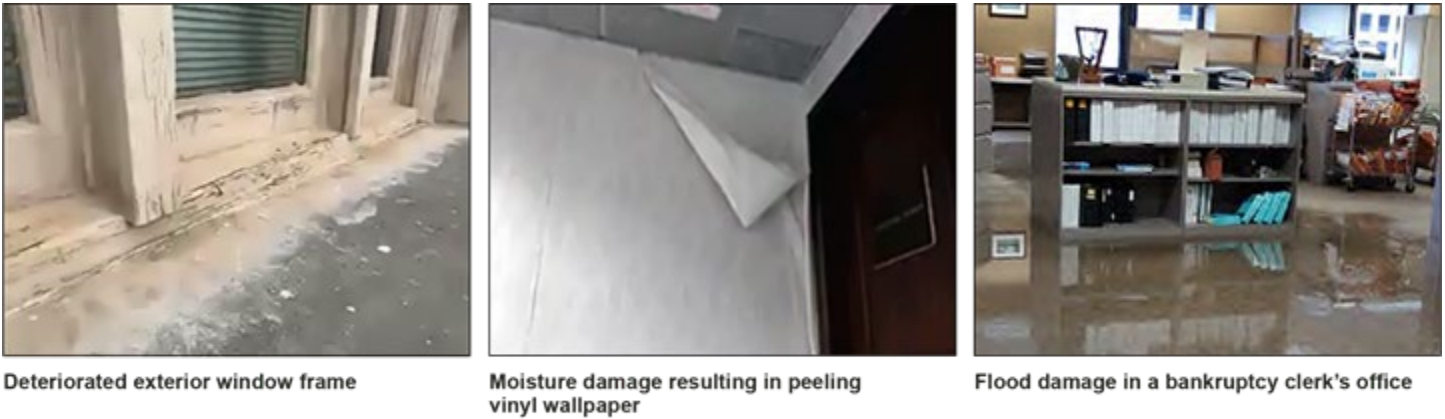
Figure 9: Depicting Courthouse General Building and Judiciary Condition Deficiencies
