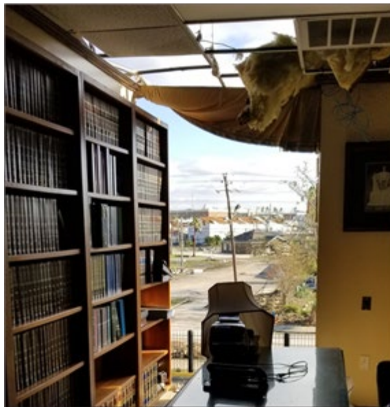
Figure 4: A Law Library at the Federal Courthouse in the Panama City, Florida, Shows Severe Damage to the Roof, Windows, and Exterior Walls After a Hurricane
