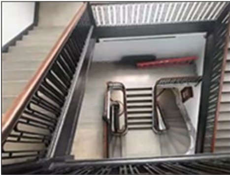
A staircase that does not meet accessibility requirements in a historic courthouse
