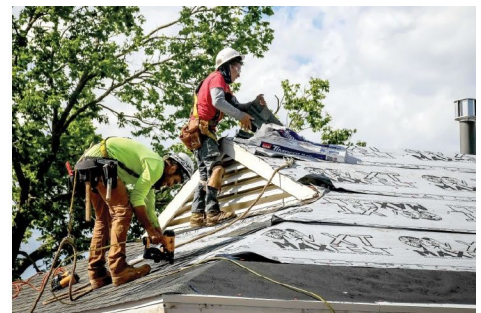
Fort Carson, Colorado (2017 / 2018) Damage from wind and hail storms
