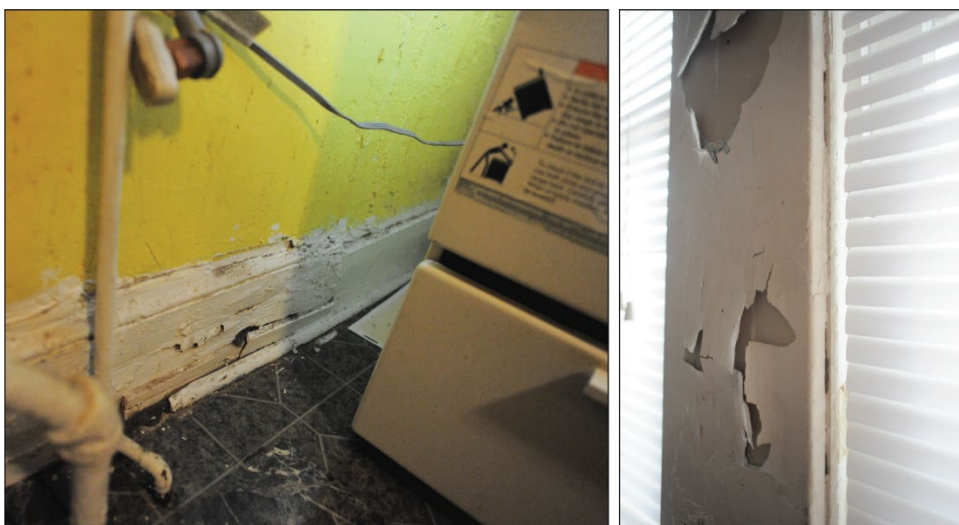
Figure 3: Examples of Deteriorated Paint
