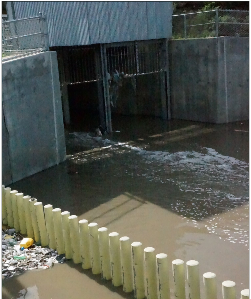
Figure 8: Trash and Sediment, South Bay Plant Canyon Collector in California
