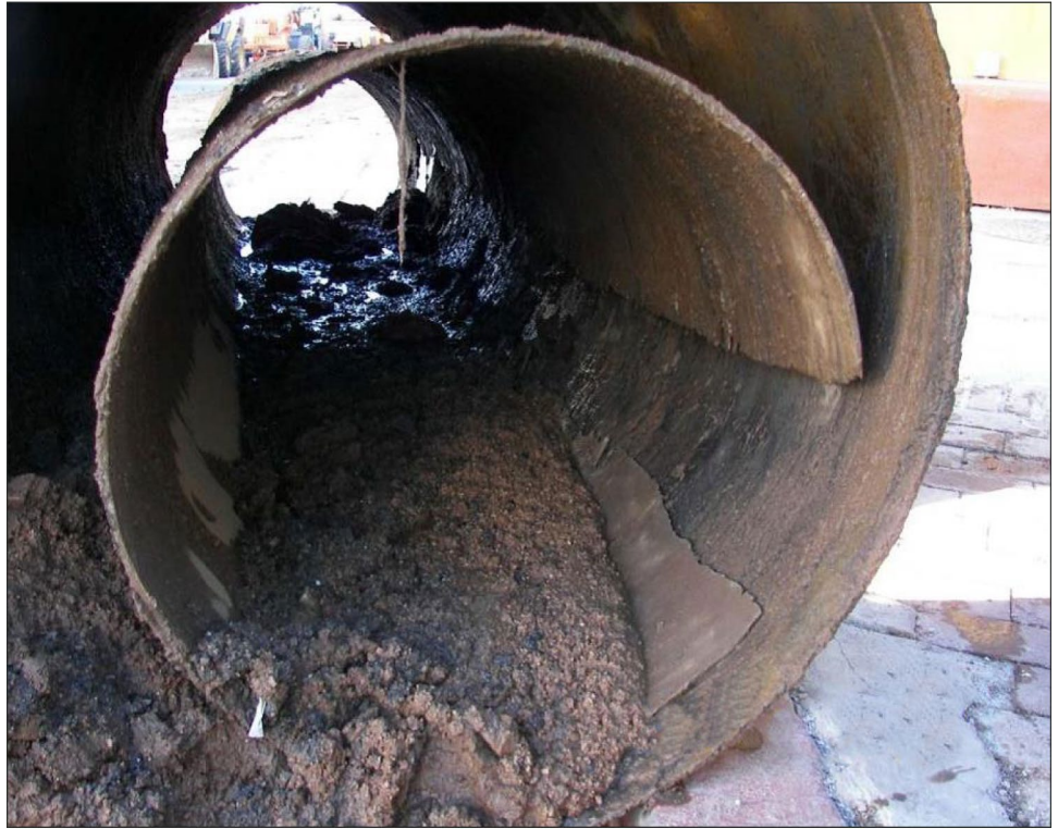
Figure 6: International Outfall Interceptor (IOI) Pipe Corrosion Due to Erosion
