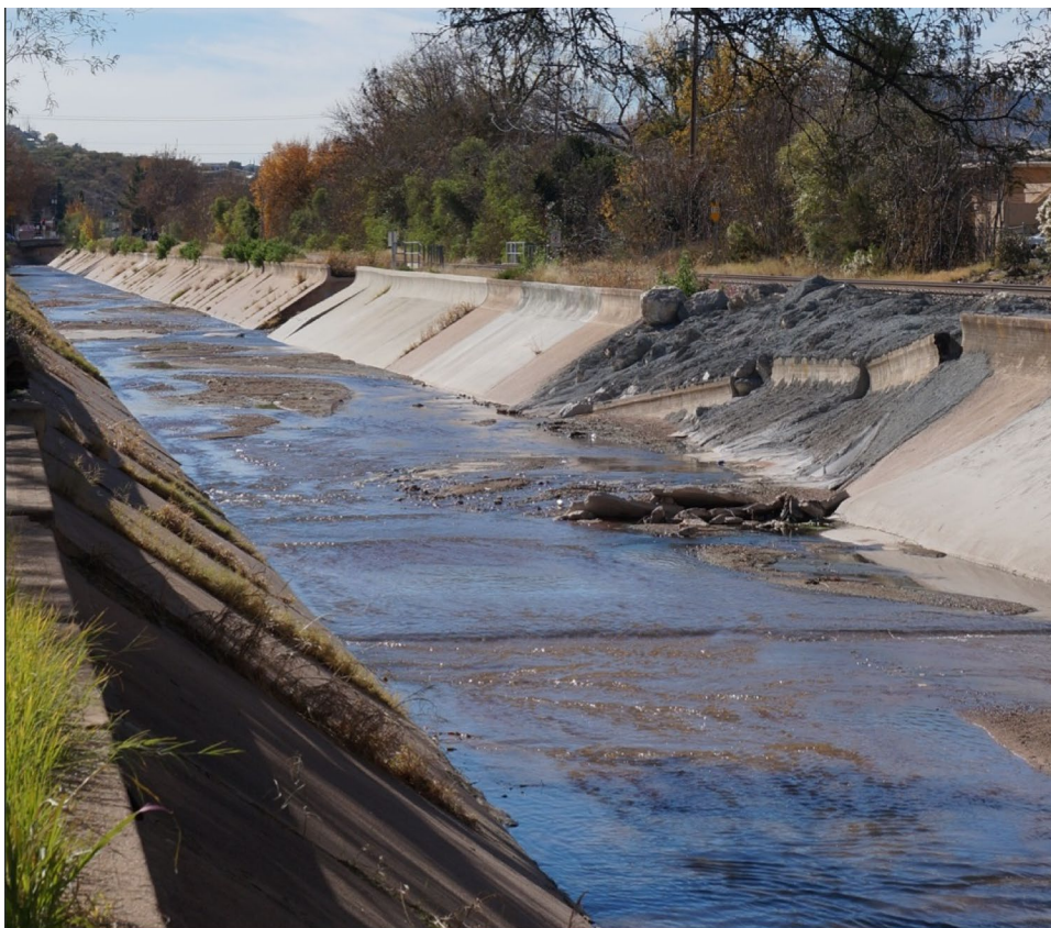
Figure 7: Collapse of Cement Panels in the Nogales Wash in Arizona
