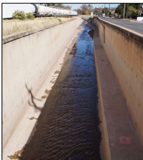
2nd Section Total length = approximately 1 mile A pipeline adjacent or underneath the concrete channel of the Nogales Wash.
