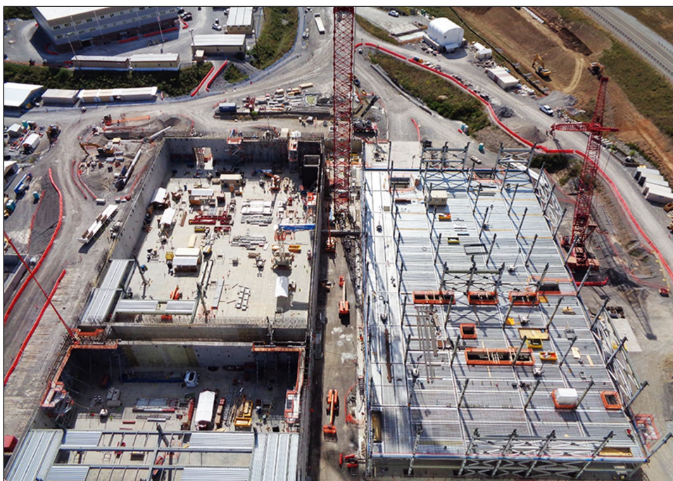
Figure 3: Ongoing Construction of the Uranium Processing Facility's Main Process Building and Salvage and Accountability Building, September 2019
