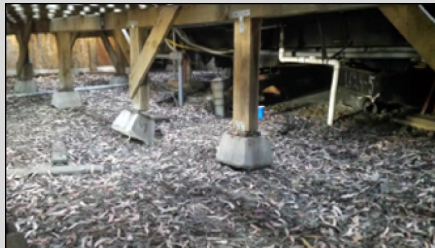
Damage to deck foundation of Station Vallejo’s main office building
