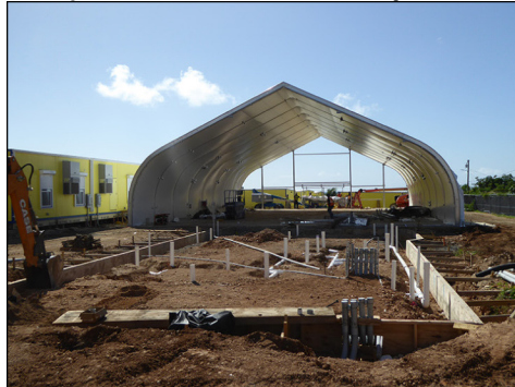
Modular units are being constructed to serve as temporary school facilities. This large unit will be the cafeteria.
