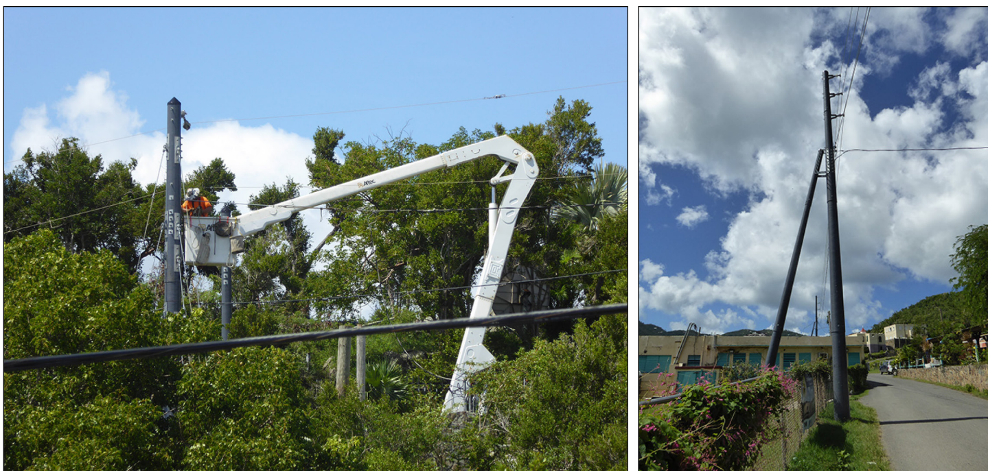
Figure 8: Composite Fiberglass Utility Poles in St. John, U.S. Virgin Islands
