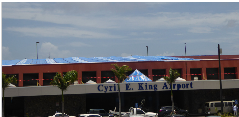
Figure 7: Roof Damage at Cyril E. King International Airport in St. Thomas, U.S. Virgin Islands
