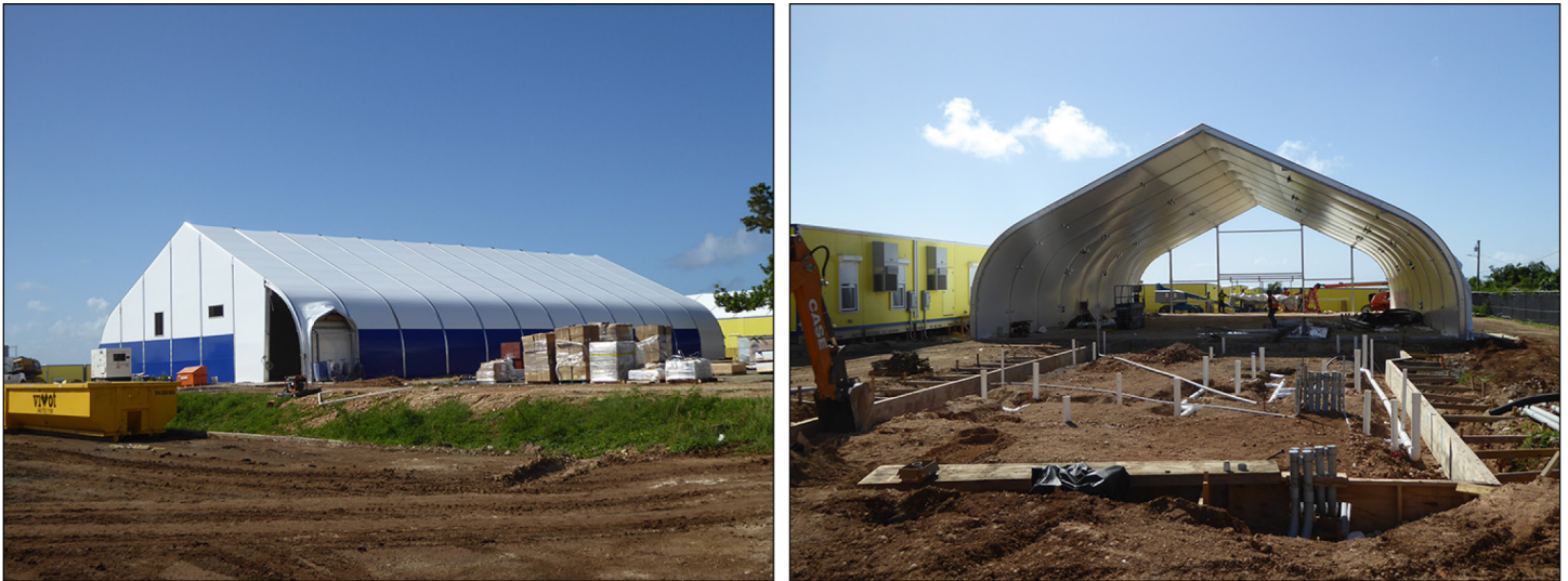
Two large modular units to provide indoor common areas, including a cafeteria.
