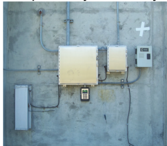
Intrusion detection systems
