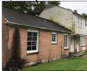
Residence hall with deferred maintenance need
