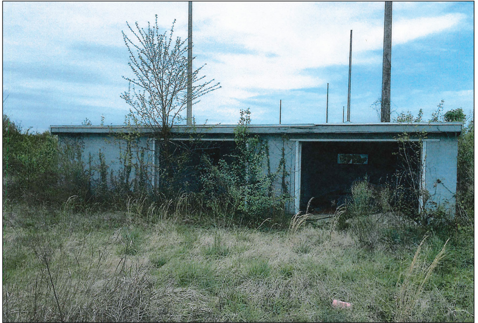
Figure 3: Abandoned Shed Found by Inventory and Recorded in the internet Navy Facility Assets Data Store as Placed in Service August 16, 2016
