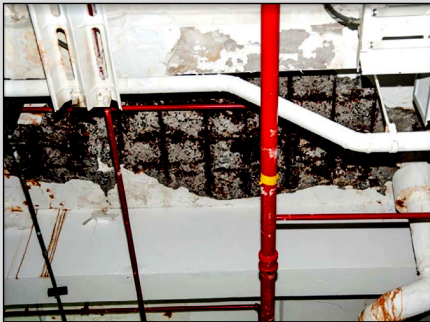
Source: Y-12 National Security Complex. | GAO-15-499
