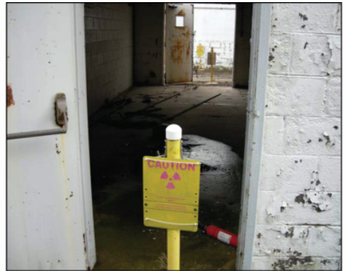
Warehouse with radiological contamination.
