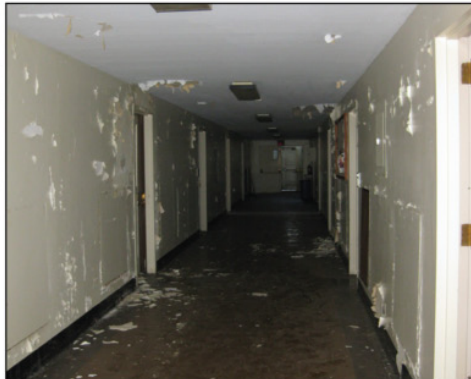
Mostly vacant laboratory building with ceiling and wall damage.
