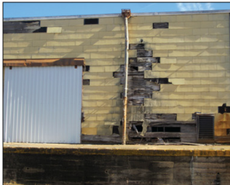
Warehouse with exterior damage.
