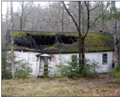
Cabin with collapsed roof.
