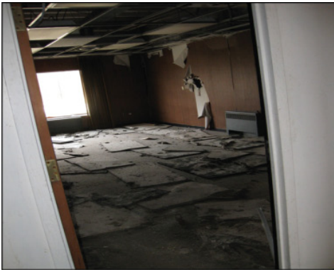
Old firehouse with collapsed ceilings.
