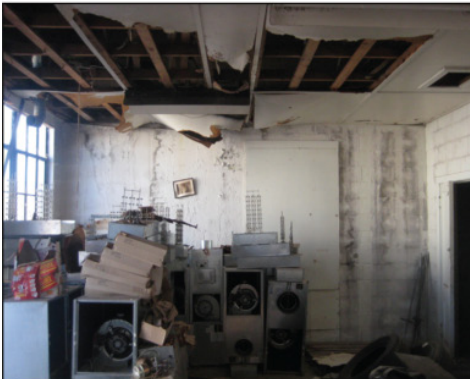
Warehouse with a collapsing ceiling.
