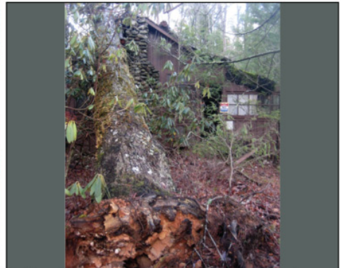
Cabin with large tree that has fallen through the roof.
