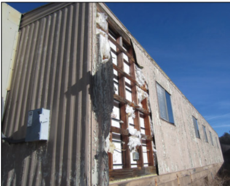
Vacant trailer with safety and health issues (rat and beehive infestation). Now demolished.
