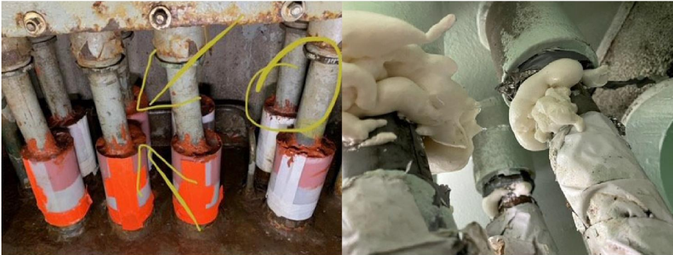
Figure 11: Use of Unauthorized Interventions, Including as Seen on Television Sealant Product and Plastic Wrap (left), Expanding Foam, Tape, and Common Store Bought Super Glue (right) as Documented by the Navy
