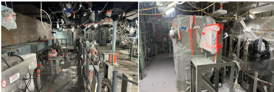
Figure 17: Incomplete Cabling and Electrical Distribution on USS Vicksburg
