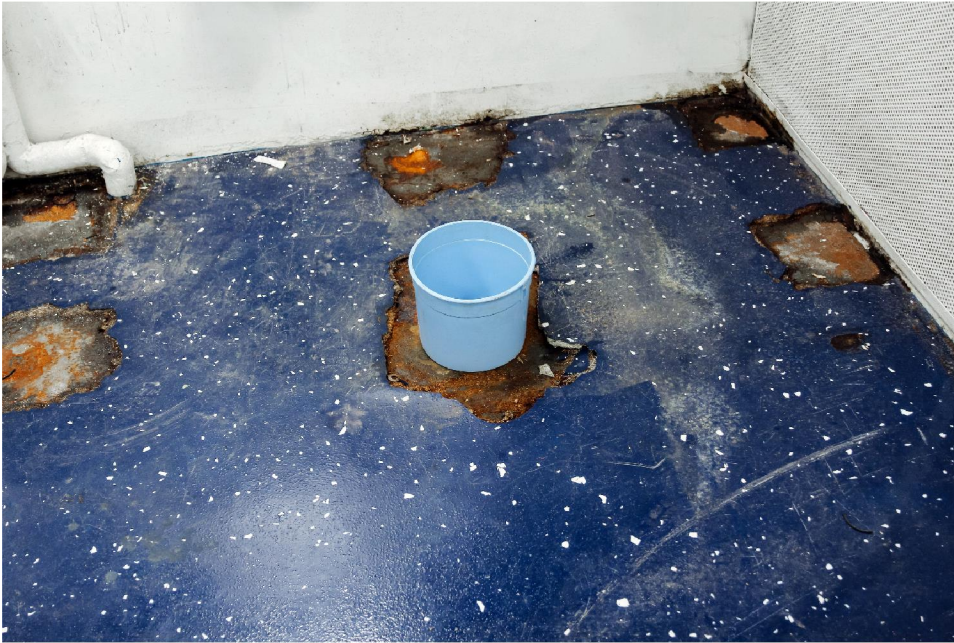
Figure 6: USS Cowpens Flooring Nearly 8 Years into Modernization
