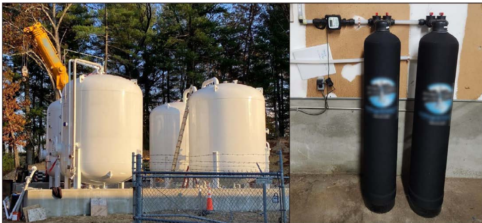
Figure 6: Examples of Granular Activated Carbon (GAC) Filtration in Large and Small Public Water Systems
