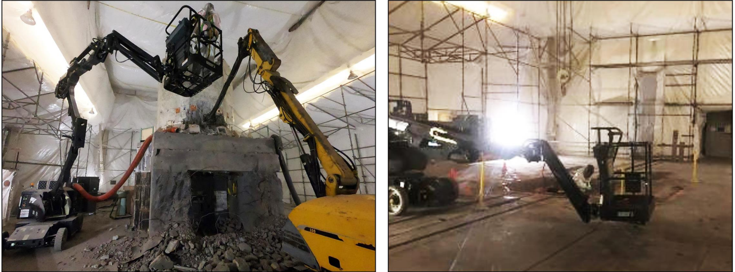
Figure 3: Deactivation and Decommissioning of the Building 280 Pool-Type Reactor at Lawrence Livermore National Laboratory
