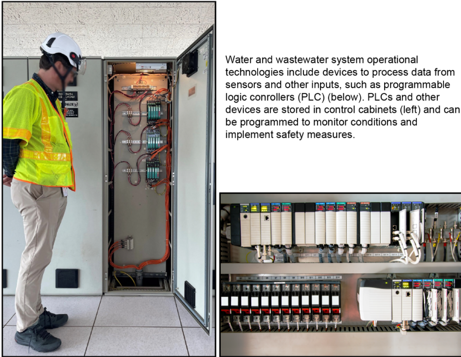
Figure 4: Examples of Water and Wastewater System Control Panels Containing Operational Technology Components
