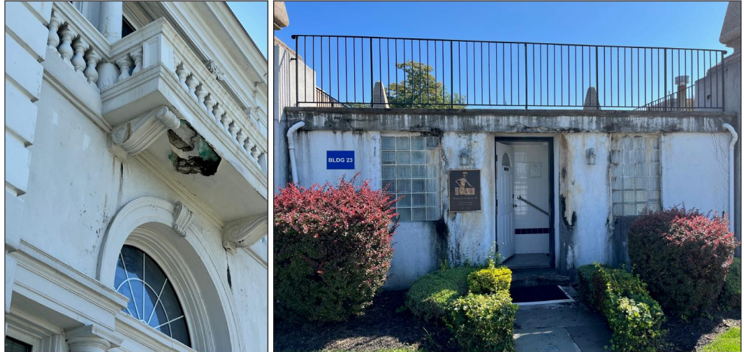
Decaying facade on Wiley Hall administration building.
