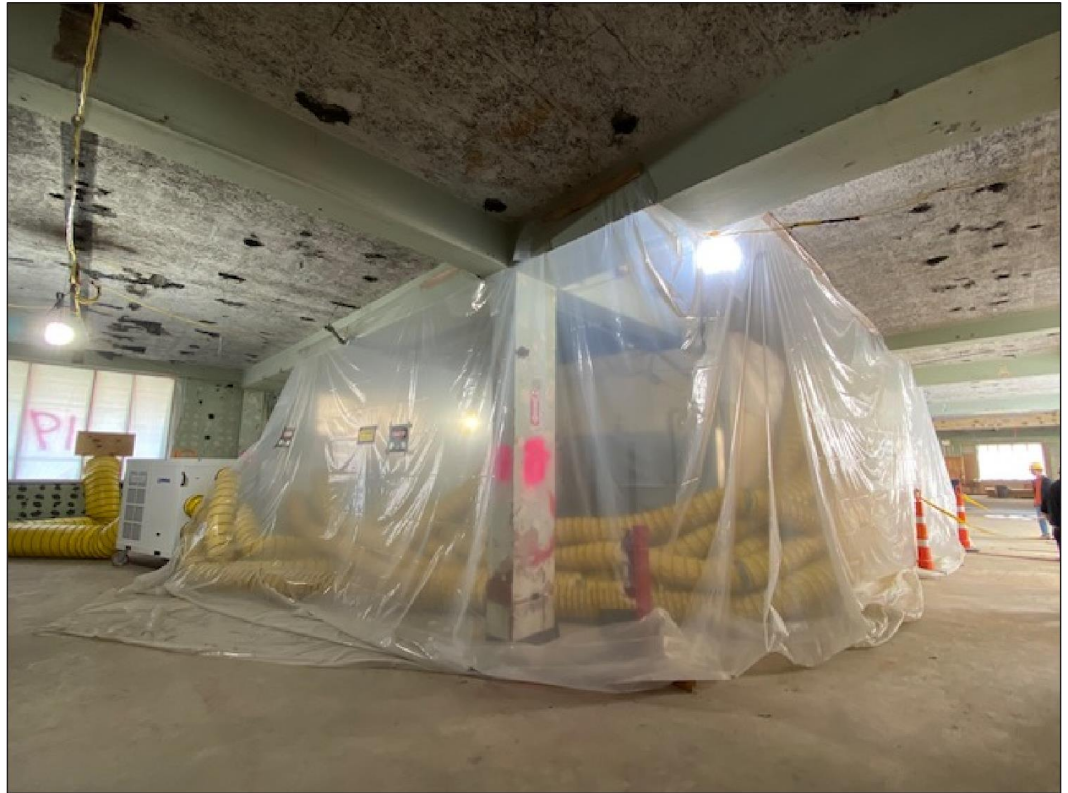
Figure 3: Samuels Hall Renovation Project, Which Includes the U.S. Merchant Marine Academy's Main Data Center, October 2023
