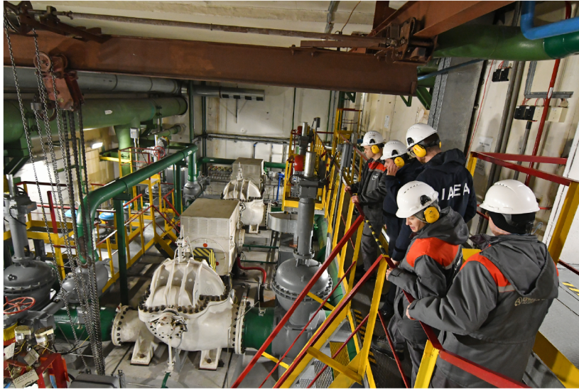
Figure 11: International Atomic Energy Agency Support and Assistance Mission in Rivne Nuclear Power Plant, Ukraine
