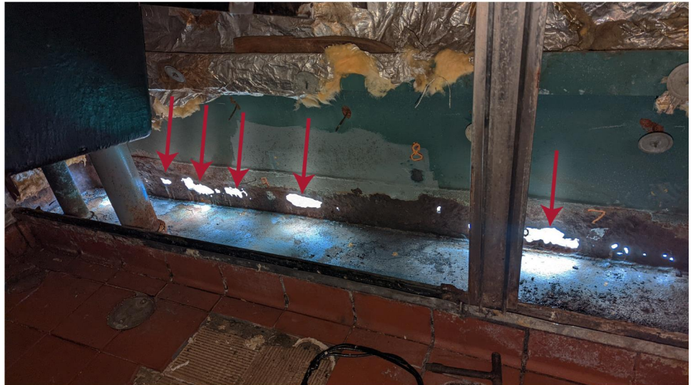
Figure 13: Corrosion through Exterior of 270-foot Medium Endurance Cutter
