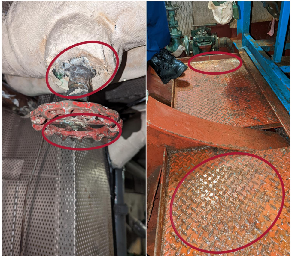
Figure 14: Condensation on Piping (left) and Corrosion on Slippery Surface (right) on 210-foot Medium Endurance Cutter (MEC)
