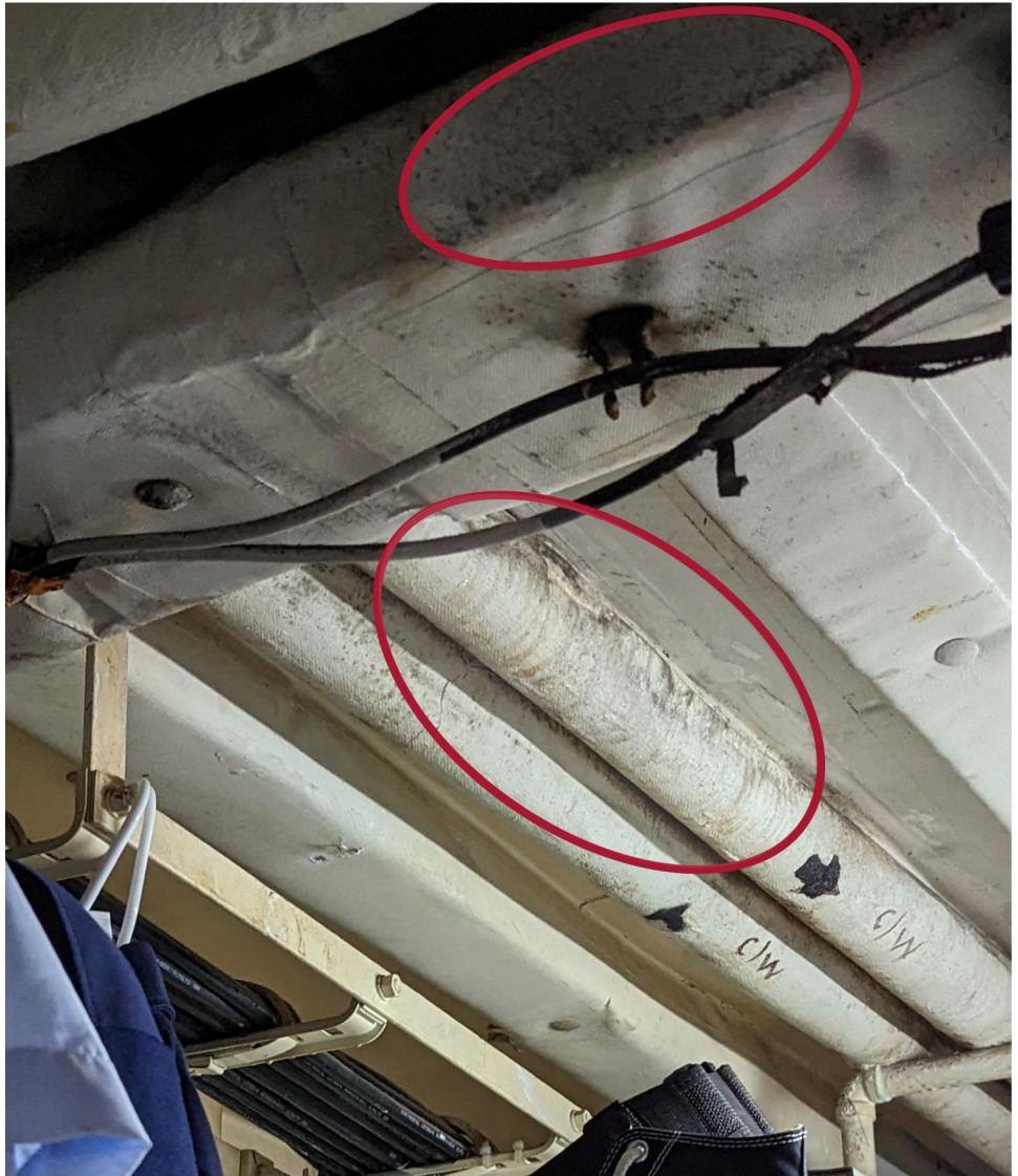
Figure 11: Mold in Berthing Area of a 210-foot Medium Endurance Cutter
