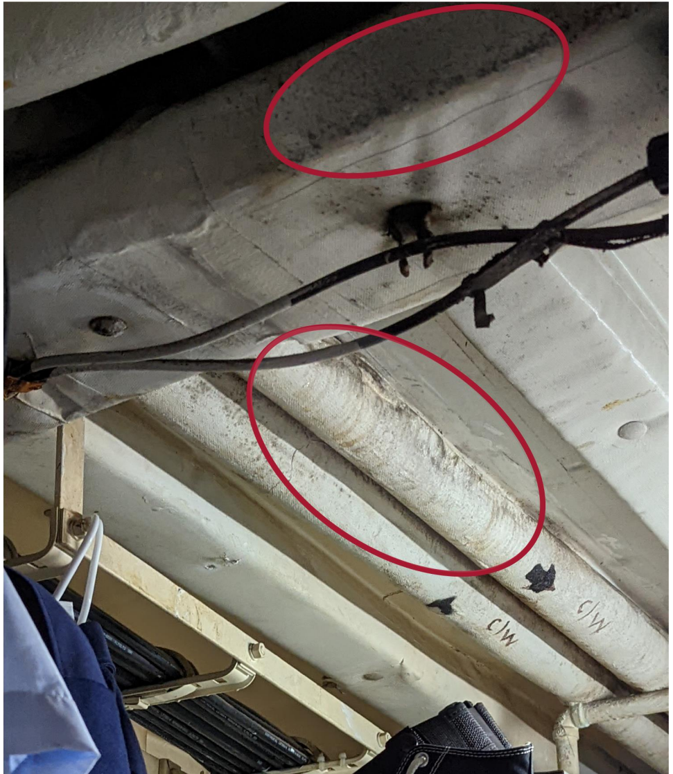
Figure 16: Mold in Berthing Area of a 210-foot Medium Endurance Cutter
