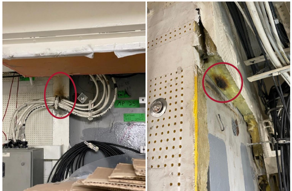
Figure 5: Damage from Two Unreported Hot-Work Incidents
