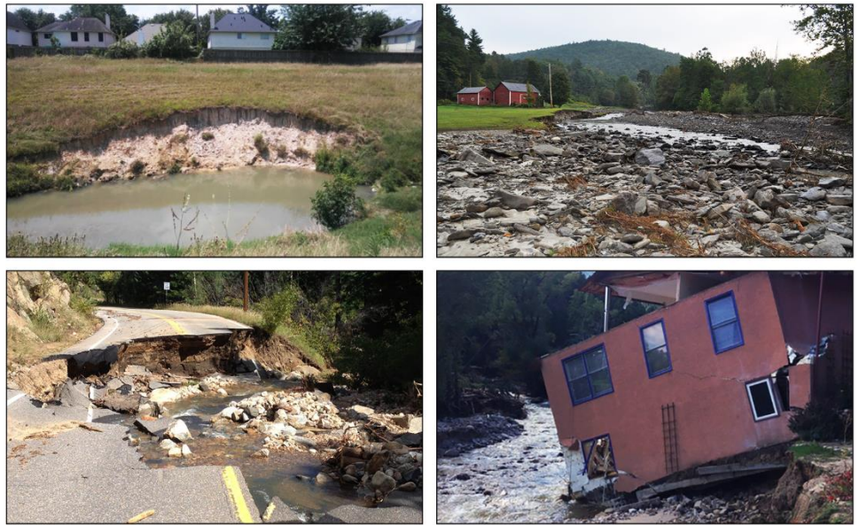
Figure 1: Flood Damage in Texas, New York, and Colorado
