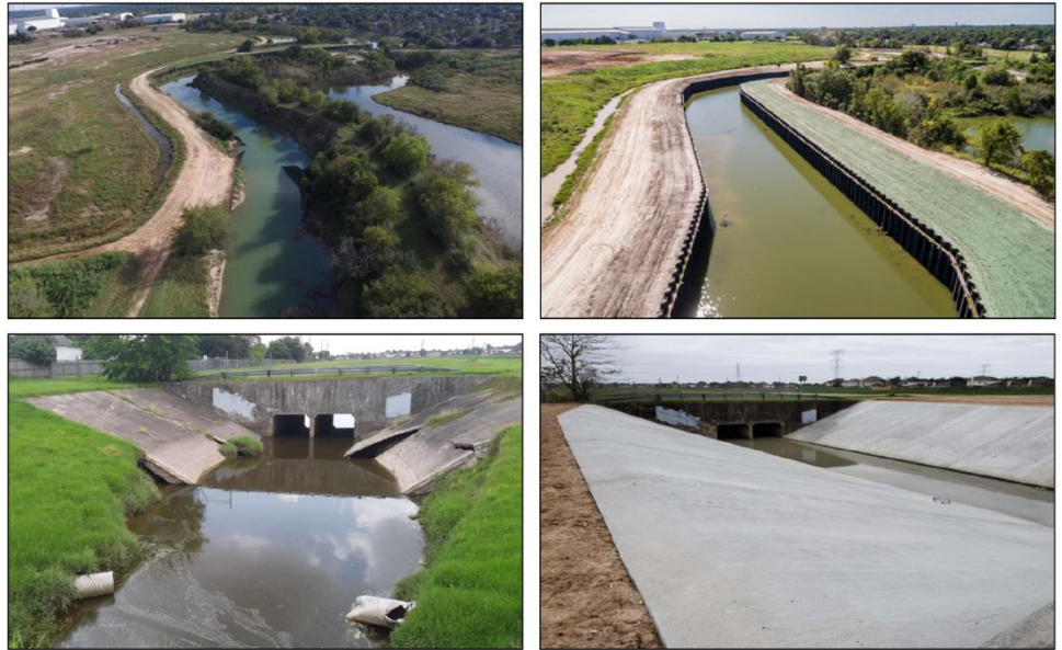
Figure 3: Post-Flood Damage and Emergency Measures in Texas
