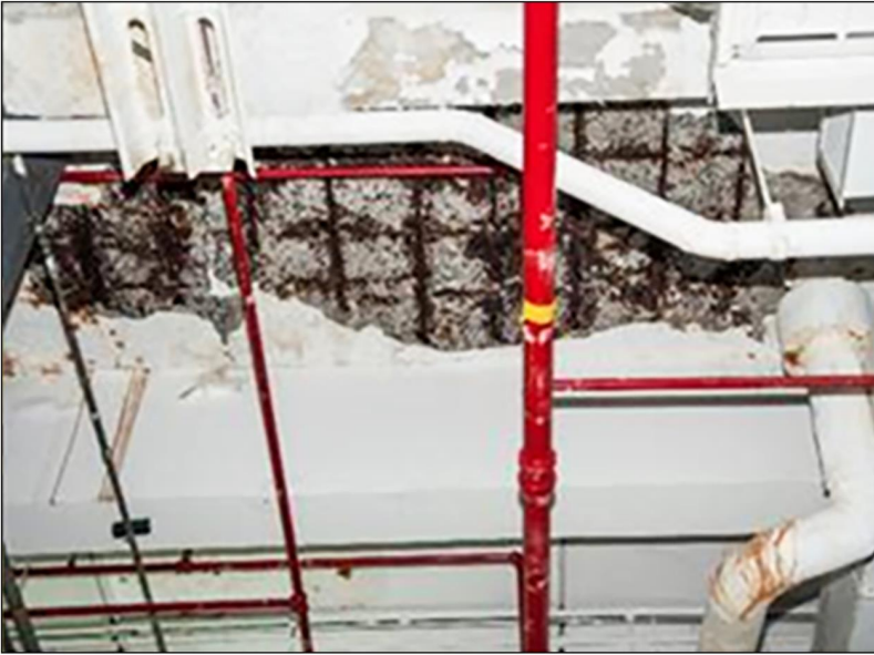
Concrete failure from 2014 on the ceiling, resulting in collapse.
