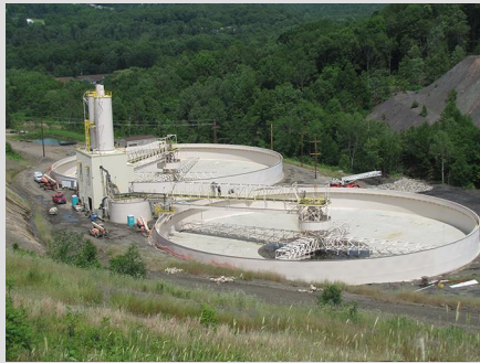
Tanks treating mining discharge at a perpetual water treatment plant.
