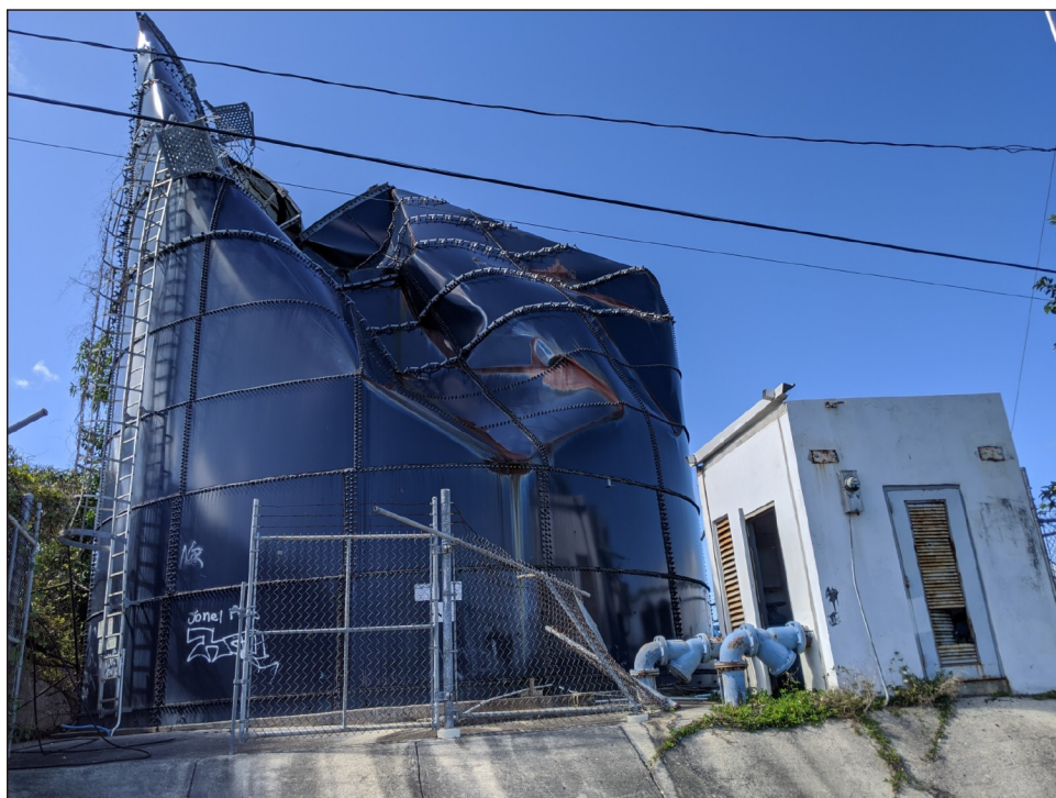
Figure 10: Damaged Water Tank, February 2020.
