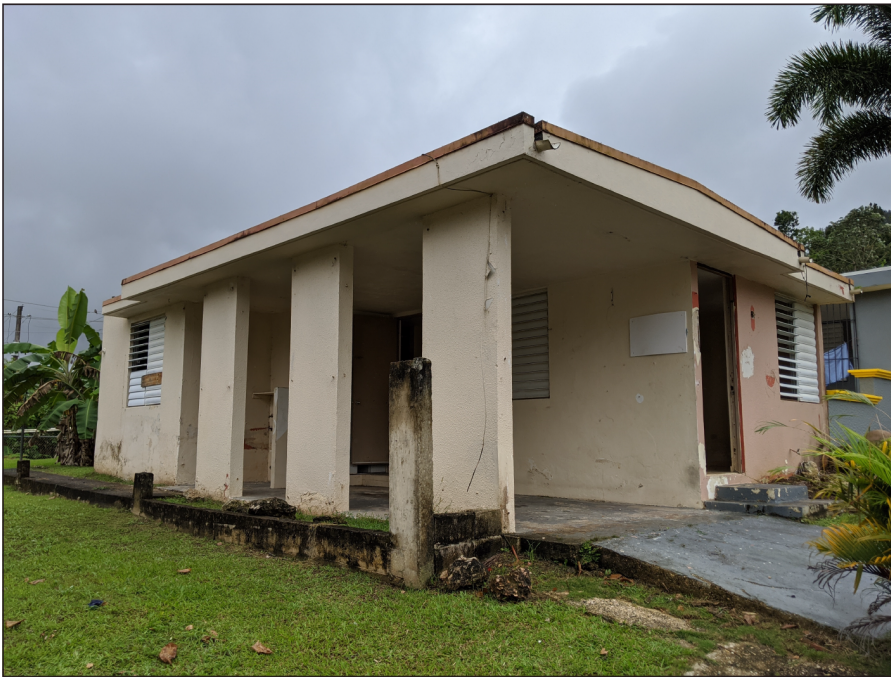
Figure 11: Damaged Public Housing units, February 2020.
