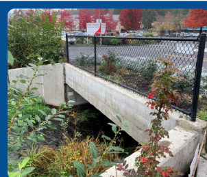
Culvert with a protective headwall that prevents erosion and allows water to pass under a road
