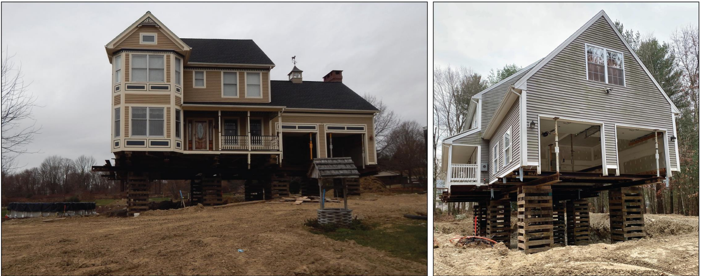
Figure 4: Homes Elevated to Replace Pyrrhotite-Damaged Foundations
