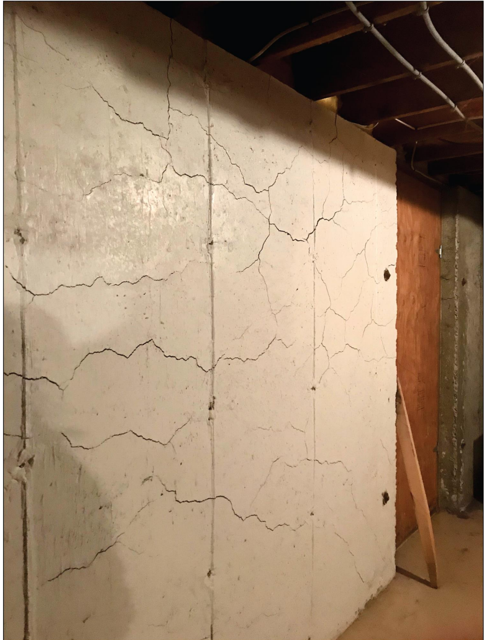
Figure 2: Basement with Severe Pyrrhotite Damage
