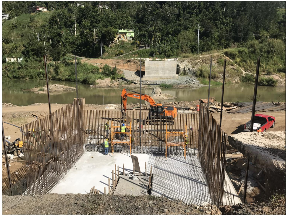
Figure 4: Initial Construction on the Ciales Temporary Bridge Emergency Repair, as of December 2018
