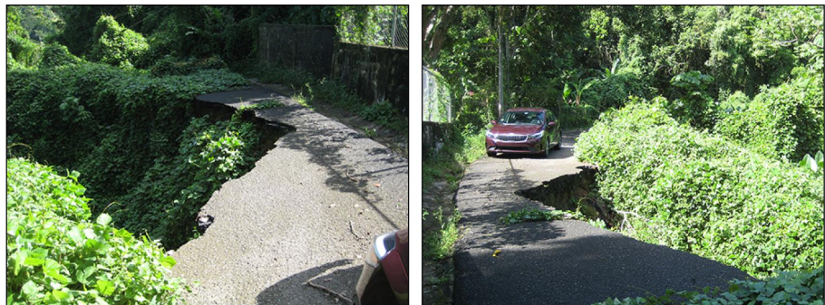
Damaged Segment of Road Near Maricao, Puerto Rico, September 2018
