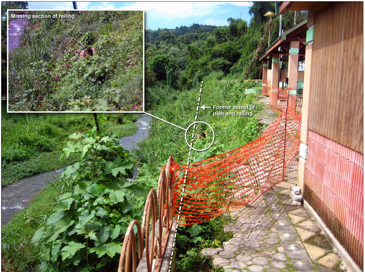
Figure 5: Missing Rail in Public Space Along River's Edge, Maricao, Puerto Rico, September 2018
