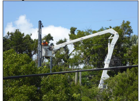
Wooden utility poles for electricity distribution are being replaced by composite fiberglass poles that can withstand 200 mile per hour winds.
