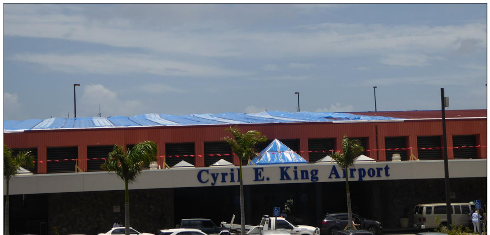
Figure 7: Roof Damage at Cyril E. King International Airport in St. Thomas, U.S. Virgin Islands
