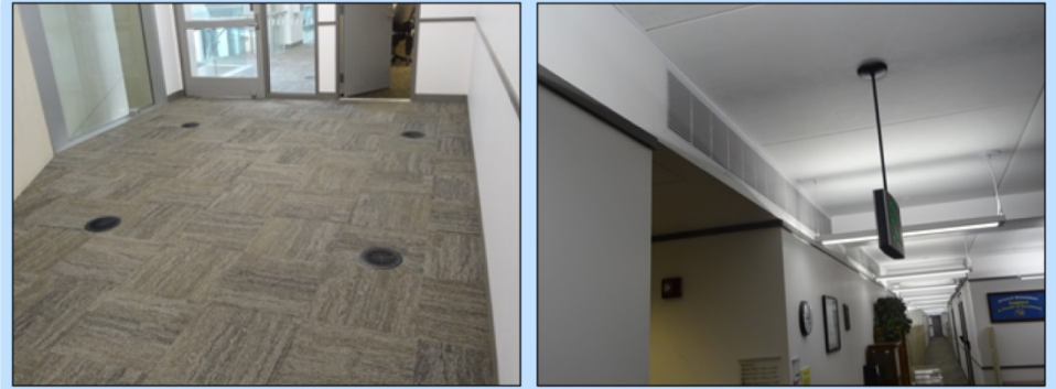
Ariel Rios Federal Building (Washington, D.C.) – The position of the building's heating, ventilation, and air-conditioning system leads to increased maintenance, repair, and energy costs. The air-supply in the raised floor (left). The air-return in the ceiling (right).
