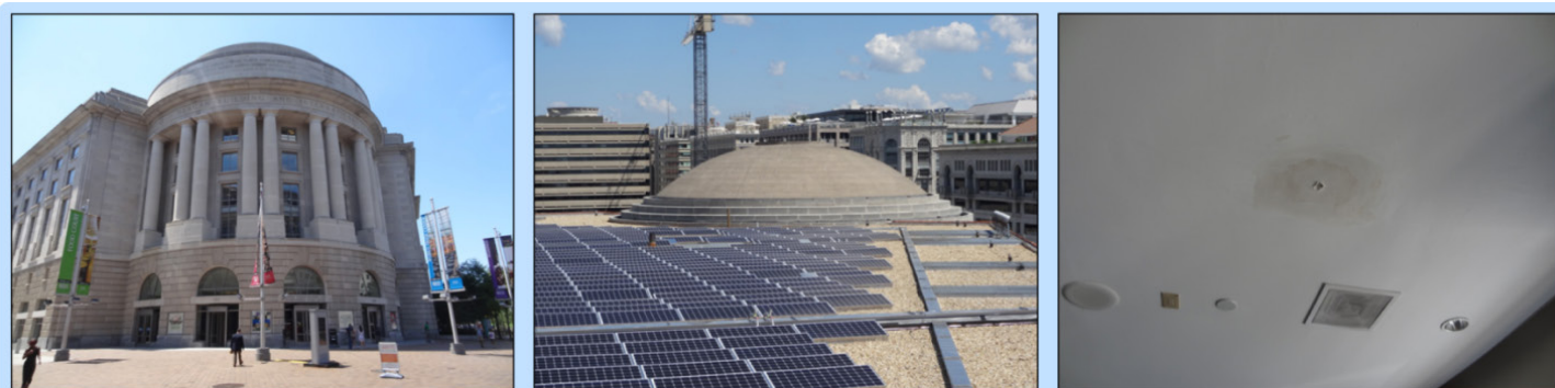
Ronald Reagan Building and International Trade Center (Washington D.C.) rotunda – Leaking gutters on the roof create water stains in the ceiling. Specialists must be hired to fix gutters because the dome roof has no area to stand.
