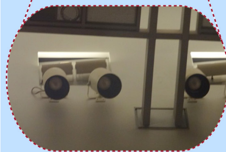
Ronald Reagan Federal Building and Courthouse (Santa Ana, CA) – Lights difficult to access and replace due to seating below and slope of floor. Requires a special equipment to replace.
