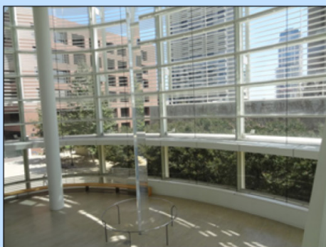
James M. Carter and Judith N. Keep U.S. Courthouse (San Diego, CA) – The atrium windows are difficult to clean due to their architectural features.
