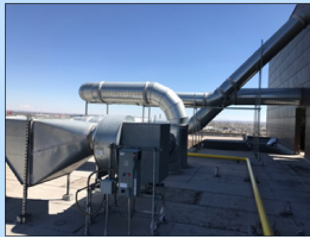
Albert Armendariz, Sr., U.S. Courthouse (El Paso, TX) – The heating, ventilation, and air conditioning chillers are located on the roof, which requires pumping water up 8 floors from the basement.
