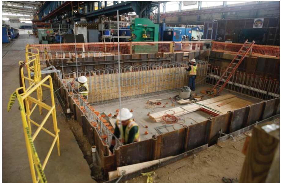
Figure 11: Foundation Being Strengthened to Accept New Capital Equipment at Norfolk Naval Shipyard
