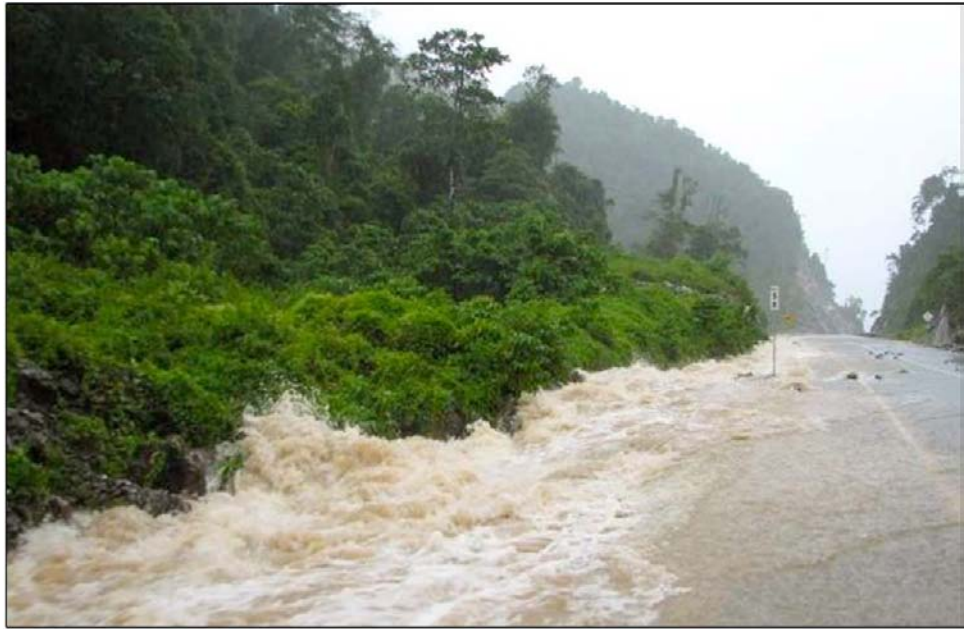
Figure 7: Flooding of Road Section Caused by Torrential Rains and Inaccurate Design
