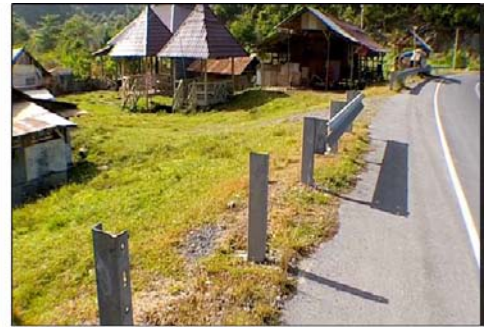
Unauthorized access road and removed guardrail
