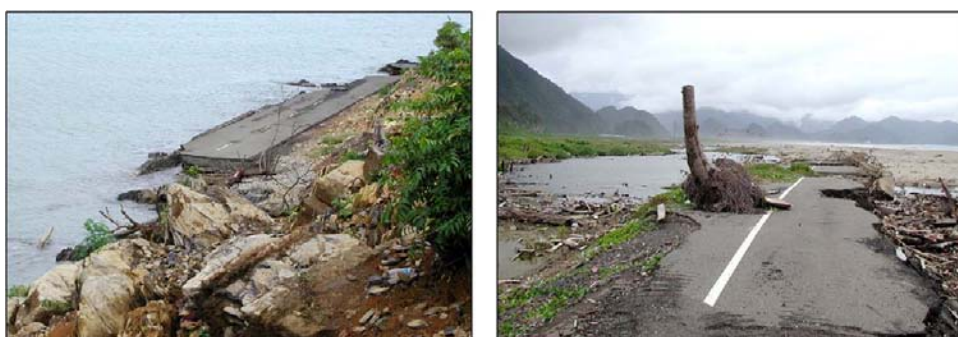
Figure 2: Destroyed Road Sections in December 2005, One Year after the Tsunami
