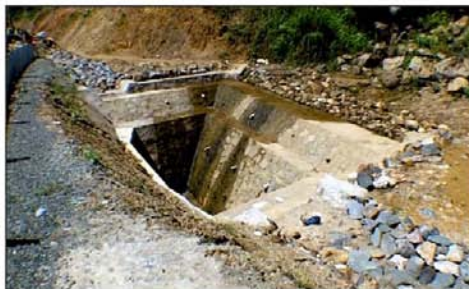
Water drainage system
