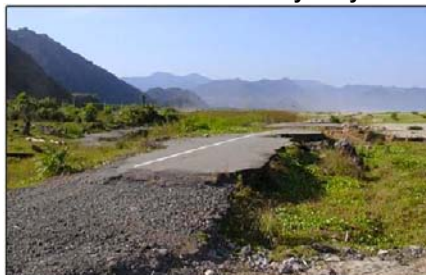
Source: GAO. Section of old road destroyed by tsunami
