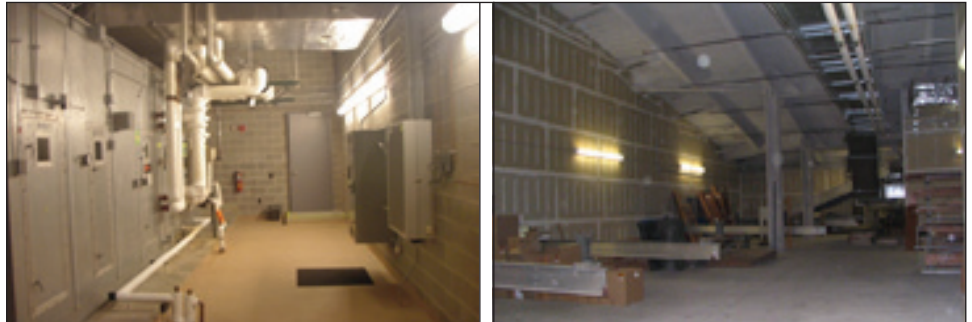
Figure 4: Example of a Mechanical Room on a Courtroom Floor of the Eagleton U.S. Courthouse in St. Louis, Missouri, and on the Top Level of the Coyle U.S. Courthouse, in Fresno, California
