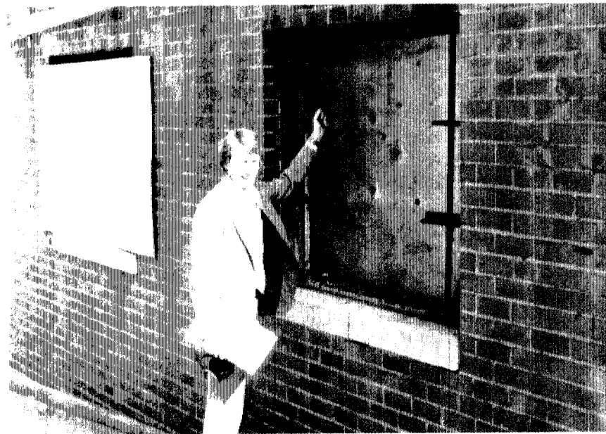
BROKEN FIRST FLOOR WINDOWS ARE COVERED BY PLYWOOD, WHICH IS EASILY REMOVED FOR UNAUTHORIZED ENTRY. AS OF MAY 1980 THE WINDOW GLASS HAD NOT YET BEEN REPLACED.
