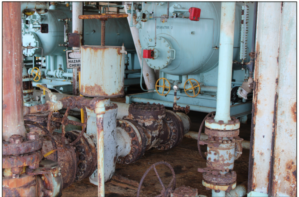
Figure 1: Corrosion on Platform Hogan in the Pacific Region
