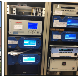
Equipment for monitoring criteria pollutants operated by the Colorado Department of Public Health and Environment
