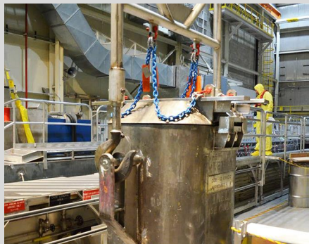
Source: Department of Energy (DOE). | GAO-23-106081
